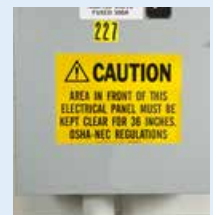
Hazard warning signs
