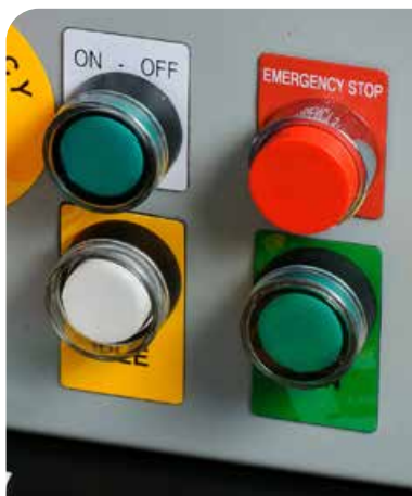
Control panel labels
