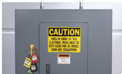
Panel & Enclosure ID
